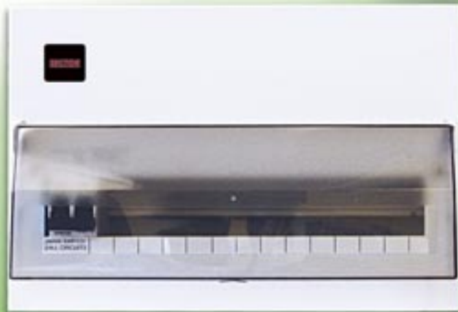
Main switch Incomer
