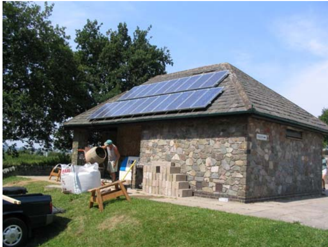
A cost effective solution - Multiple 80W solar panels installed at a park to provide lighting and automatic gate opening all year round.
